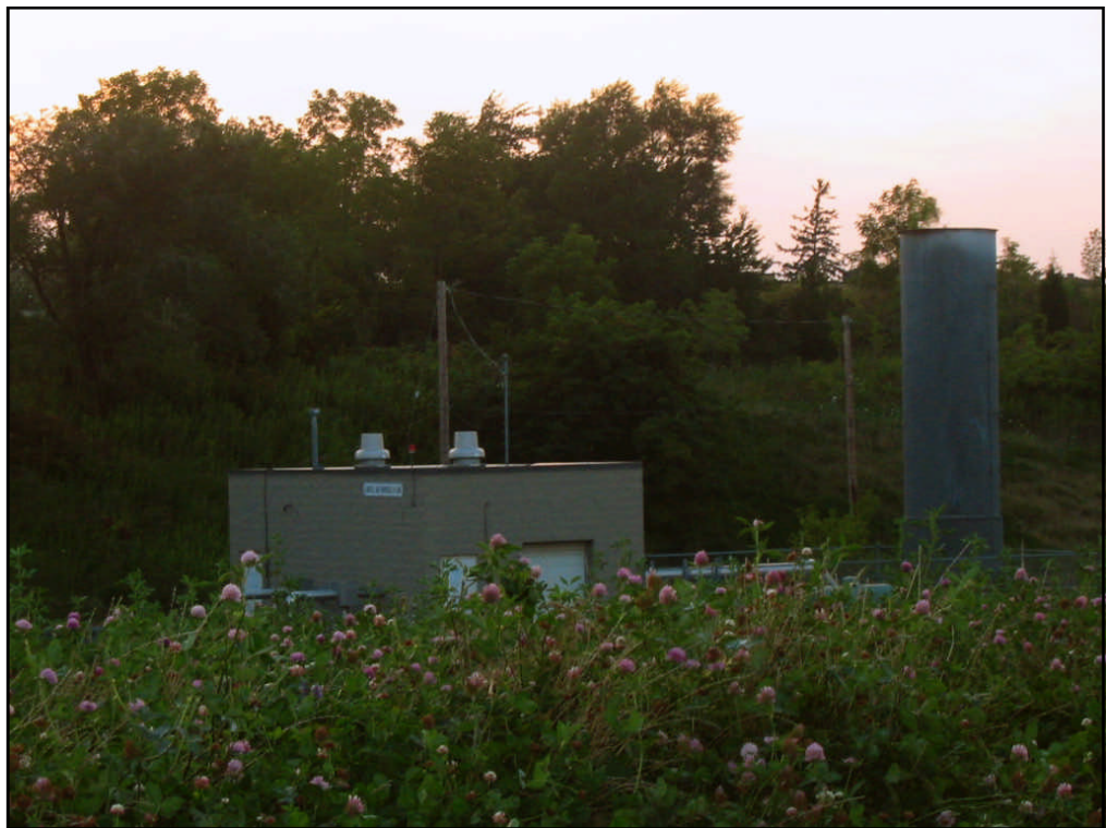
Landfill Gas Collection System at Glenridge Quarry Landfill
