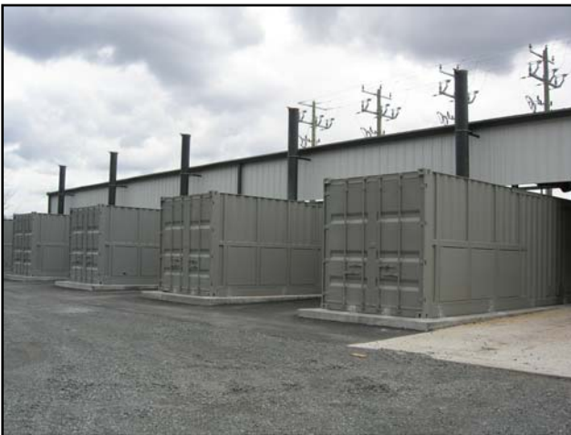
Engine/generator sets at the Trail Road Facility
