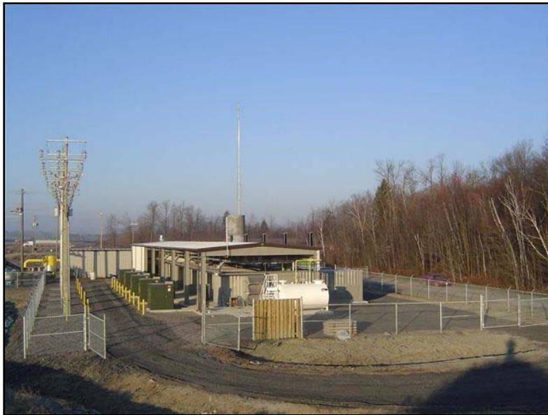
Trail Road Landfill Gas to Energy Facility
