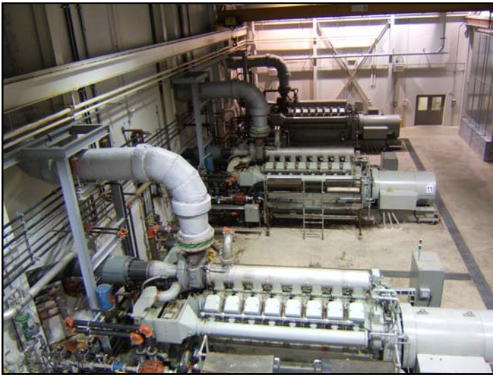
Engine/generator sets at the Britannia Landfill Gas Compression and Electrical Generation Facility
