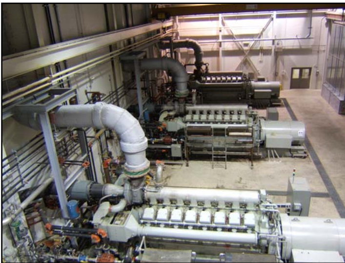
Engine/generator sets at the Britannia Landfill Gas Compression and Electrical Generation Facility
