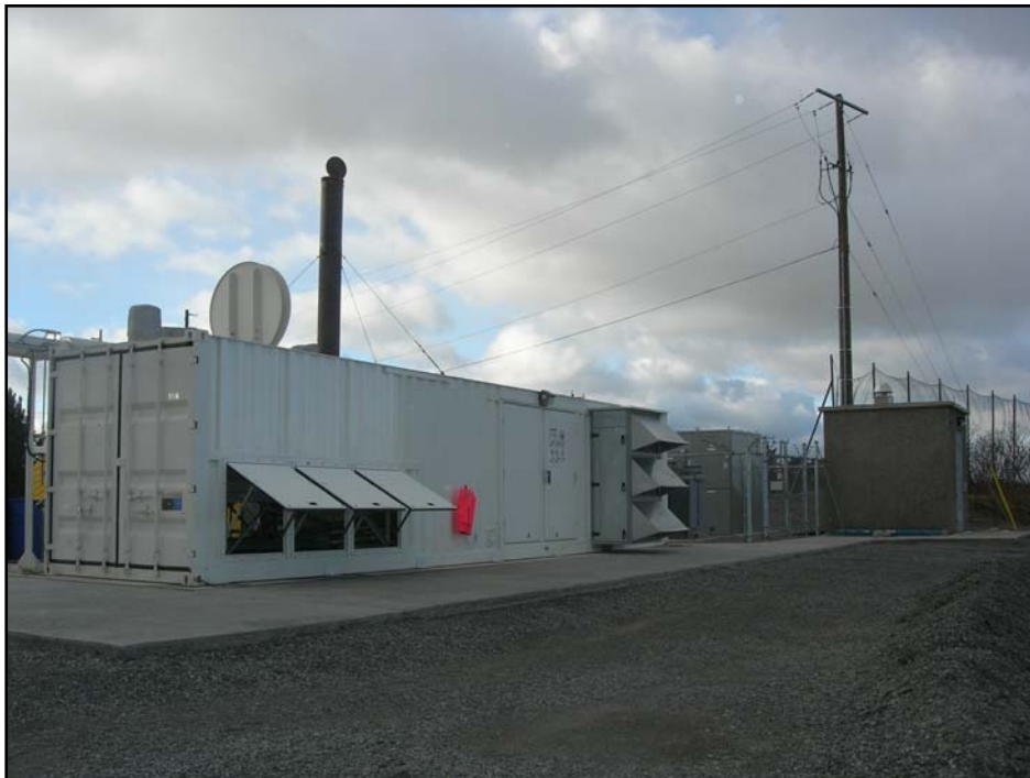
East Landfill Gas to Energy Facility
