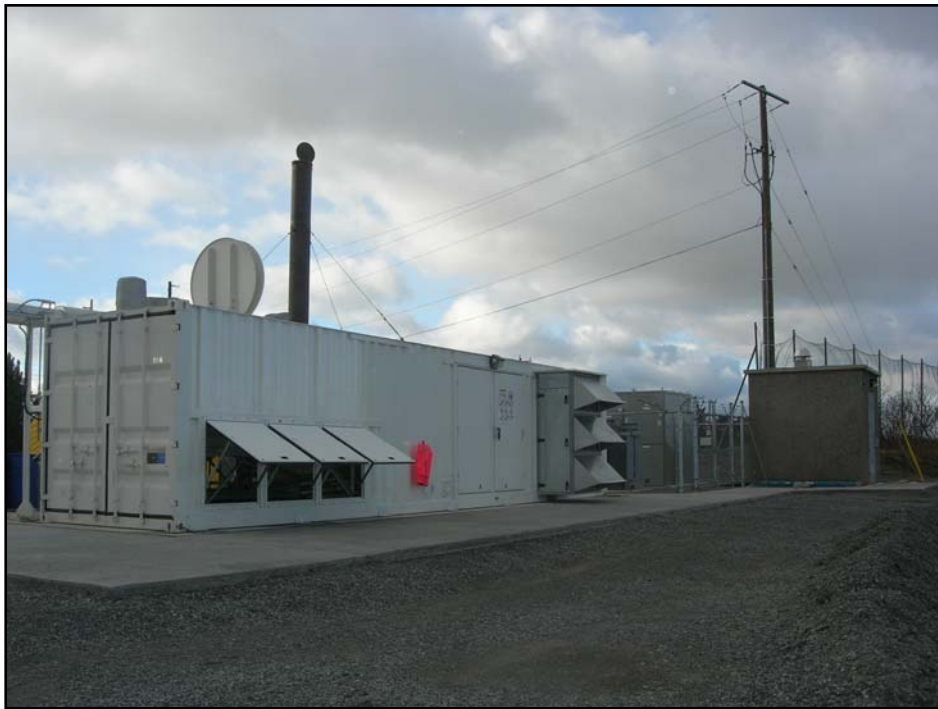
East Landfill Gas to Energy Facility
